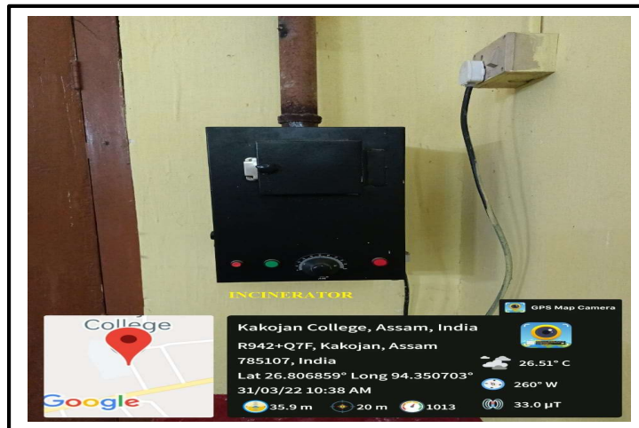
Girls' Common room sanitary pads Disposal machine
